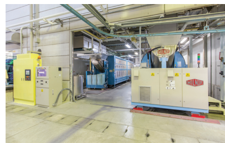
TWO GENERATIONS: The Maruwa laundry’s PulseFlow CBW tunnel (right) is seen alongside the refurbished Milnor CBW tunnel (left).
