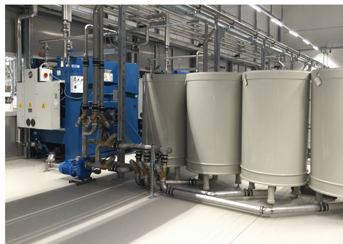
RE-USE TANKS: DBL Kuntze & Burgheim uses a complex water recovery system at its laundry in Hermsdorf
