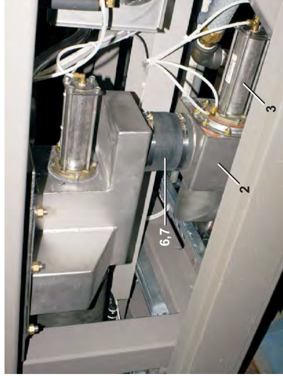
(C) Drain Stop: Flow Not to Sewer
