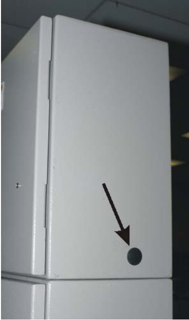
Figure 3: Hole in Shuttle Processor Box for Cable
