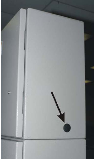
Figure 3: Hole in Shuttle Processor Box for Cable
