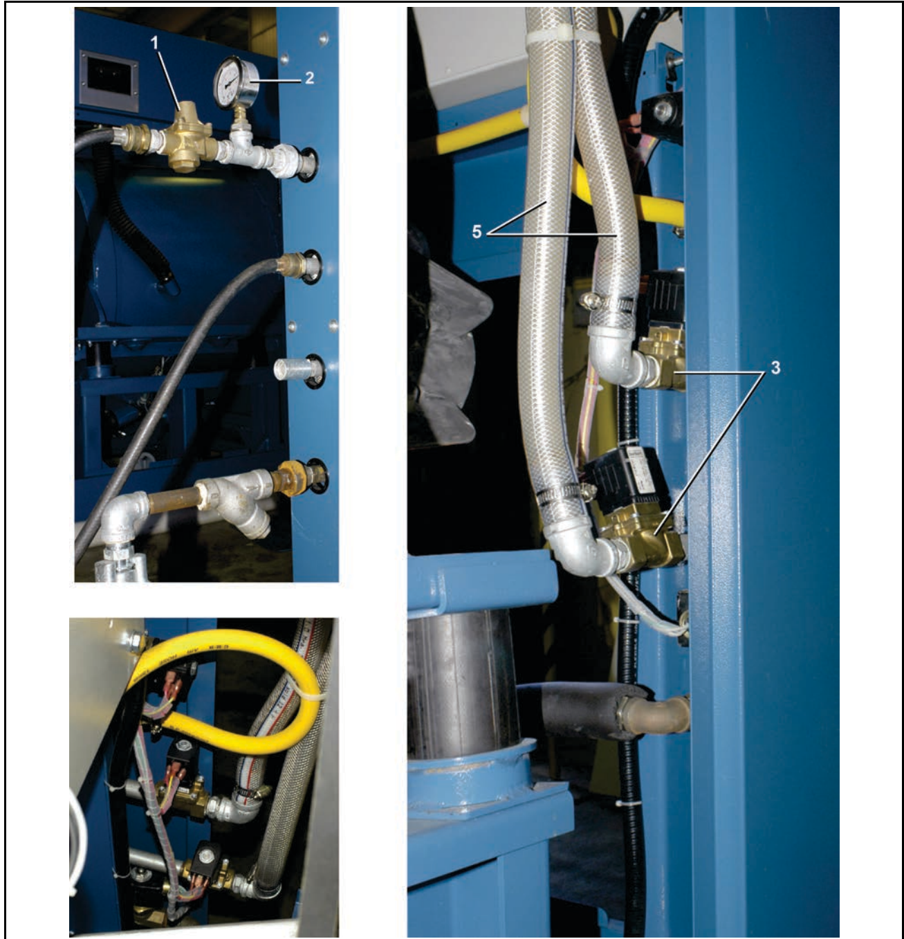
Figure 37. Water and Steam Inlets
