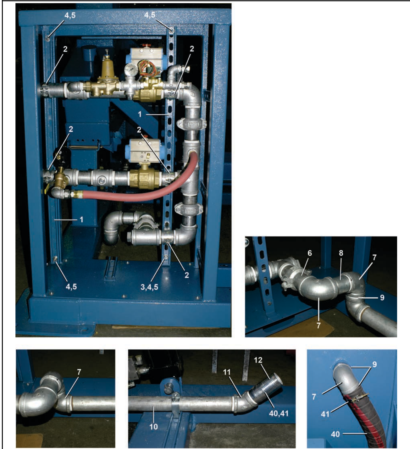
Figure 54. Water Valves Installed
