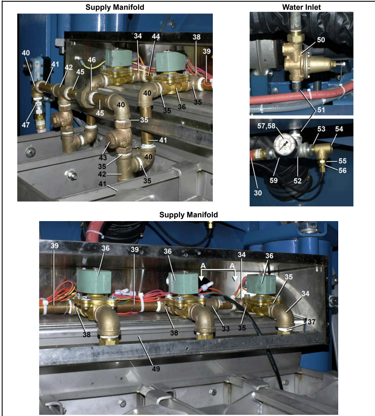
Figure 68. Water inlet and manifold piping
