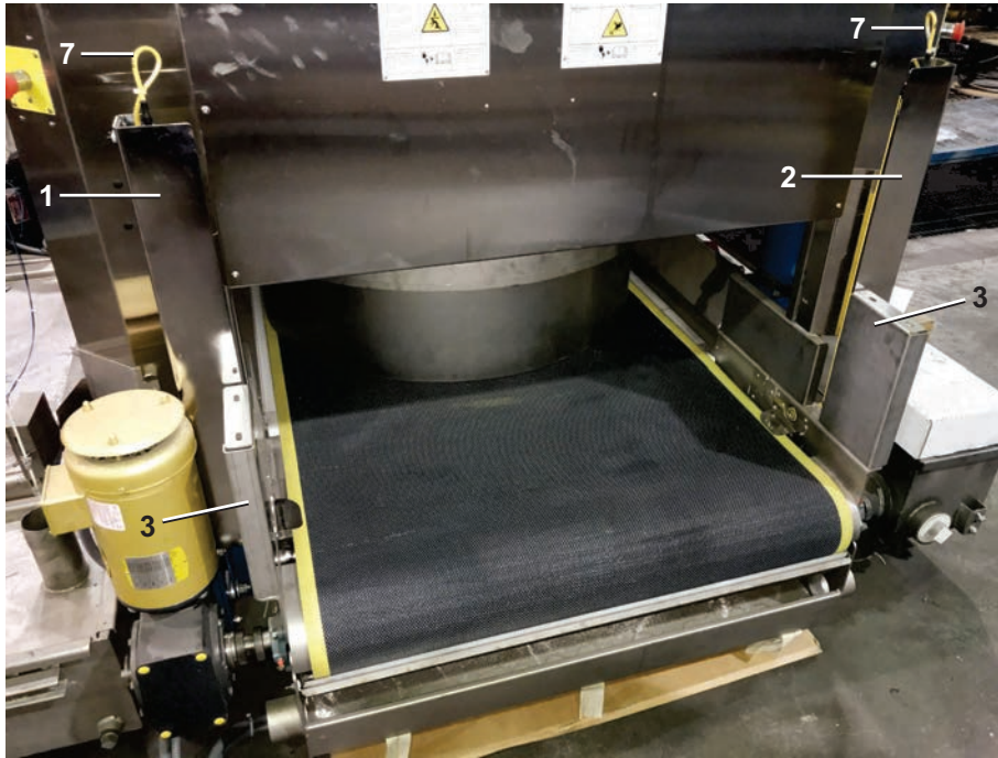
Figure 1: Emitter and Receiver Installation
