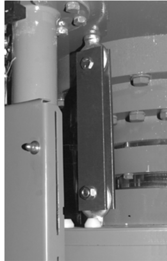
Figure 1. Safety Bars Deployed
