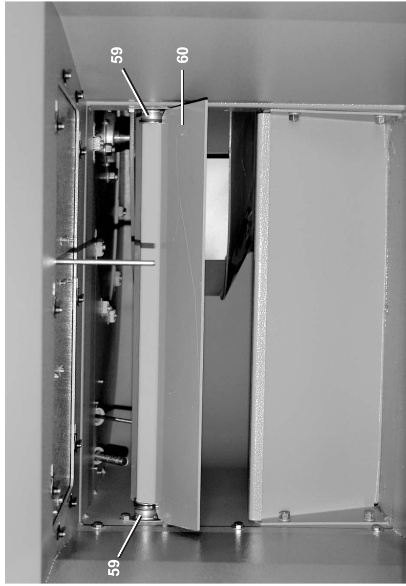
BLOWER EXHAUST DUCT
