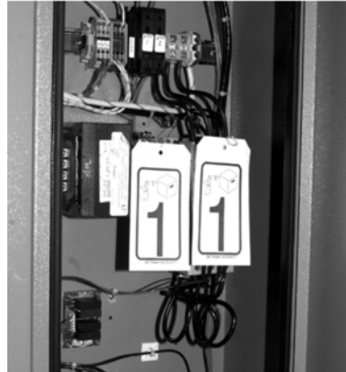
Figure 2. Reconnect Blower Contactor Coil Wires
