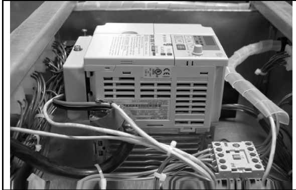
Figure 2: Inverter maintenance points (MCR18E7 shown)
