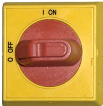
Figure 2: Motor Disconnect Switch
