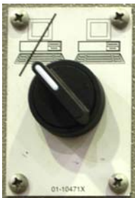
Figure 6: Mildata/Local Selector switch
