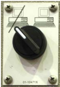
Figure 6: Mildata/Local Selector switch
