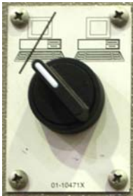
Figure 6: Mildata/Local Selector switch
