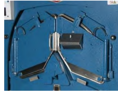
Figure 5. Rapid Load Doors
