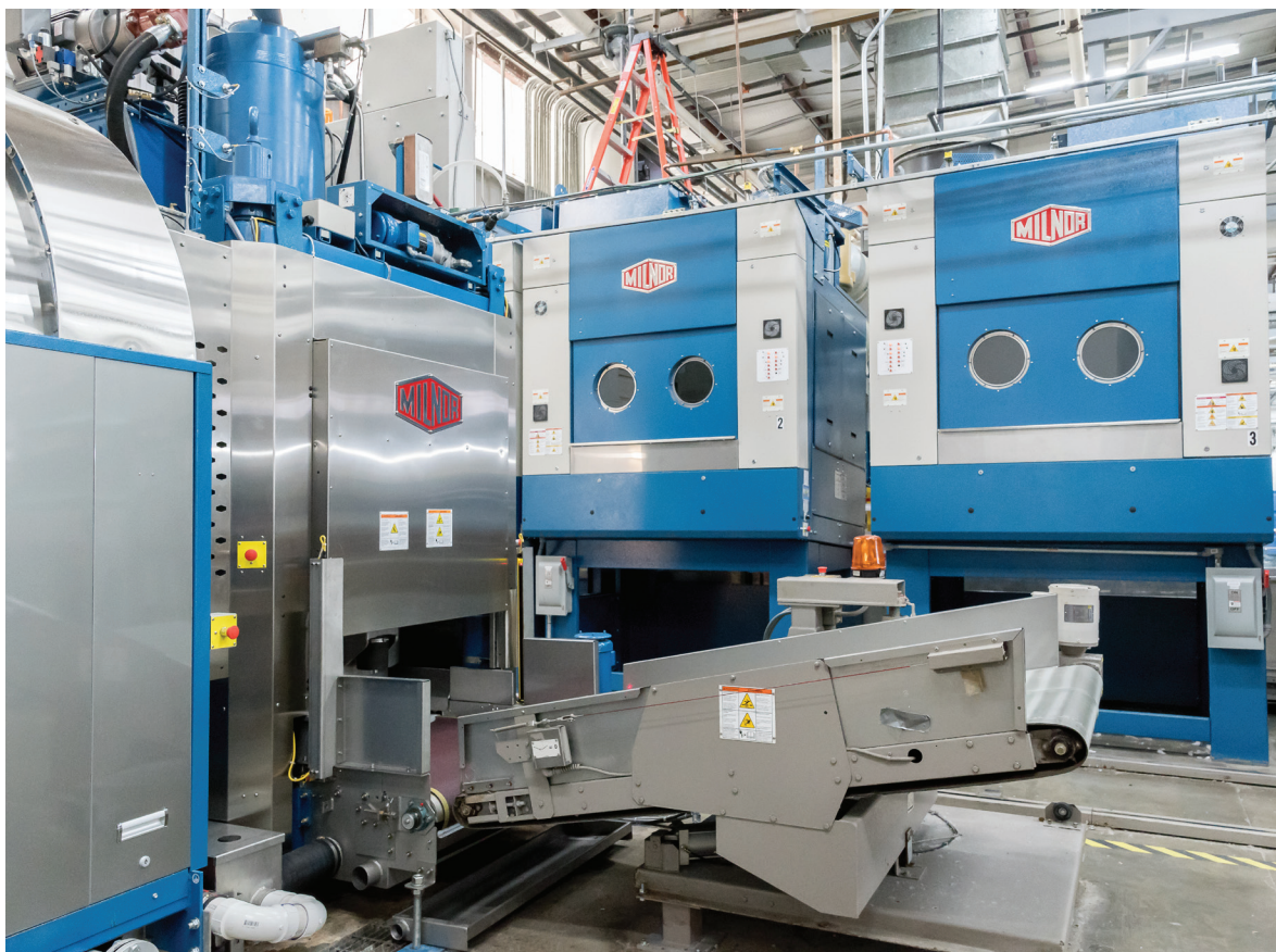
ABOVE: A view of Westport Linen Services' recently refurbished wash aisle in Baton Rouge, including a new CBW and 50 bar press that's helped this healthcare operator increase throughput, while cutting water consumption from 1.65 gal per lb. to 0.8 gal/lb.
