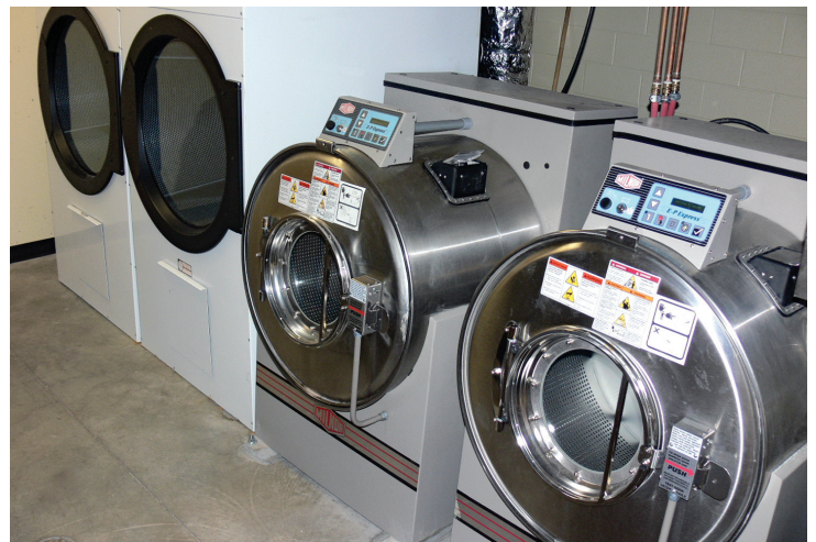
Birmingham-Southern's football facility includes two washer-extractors and two dryers, all from Pellerin Milnor Corp.
