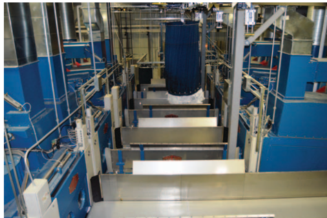
PRESS-TO-DRYER TRANSPORT: The E-Tech rail system is seen here delivering washed and extracted linen to the dryers
